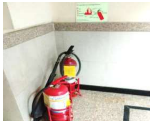
FIRE EXTINGUISHER ON EVERY FLOOR
