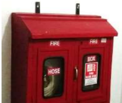
FIRE HOSE ON EVERY FLOOR
